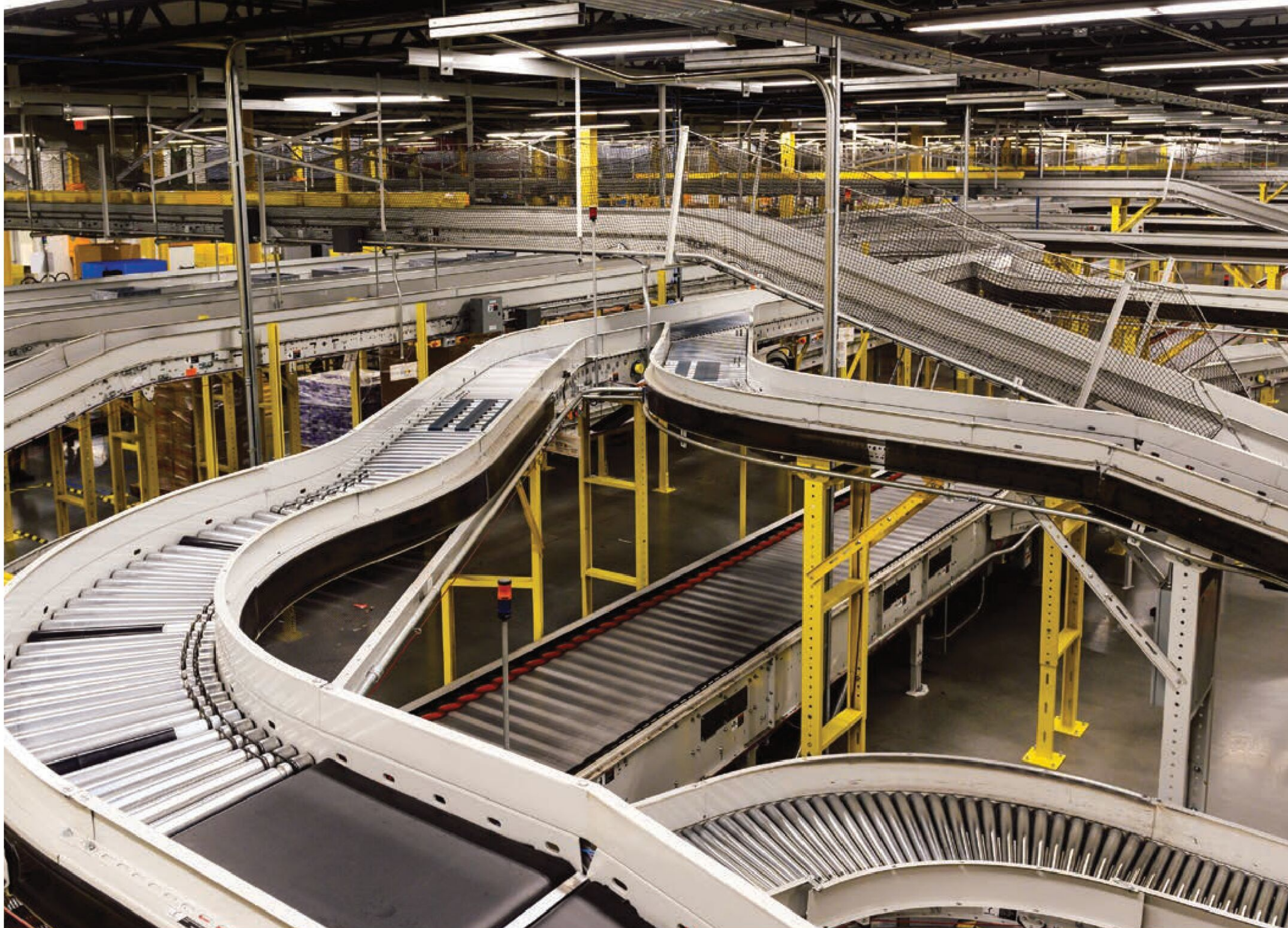
▲ A system of conveyor belts at BFI4
